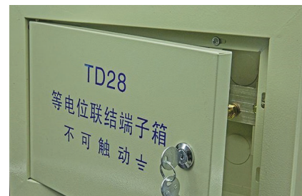
Fig. 5. Original image of power cabinet door.
